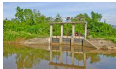
The water gate keeps fresh water for farming in dry season and to release water whenever the area is flooded. However, all water gates can't protect farming land of the community if the area is flooded by heavy rain.
